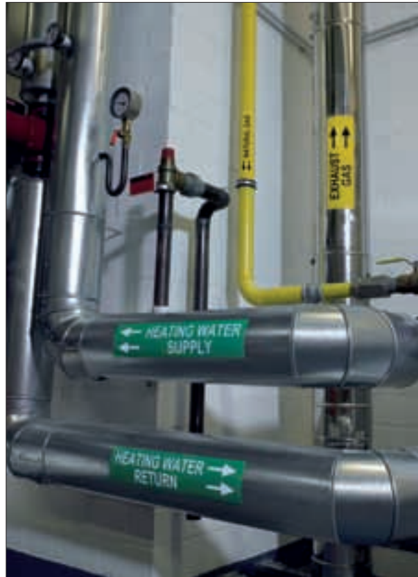
Large and highly visible pipe marking.
