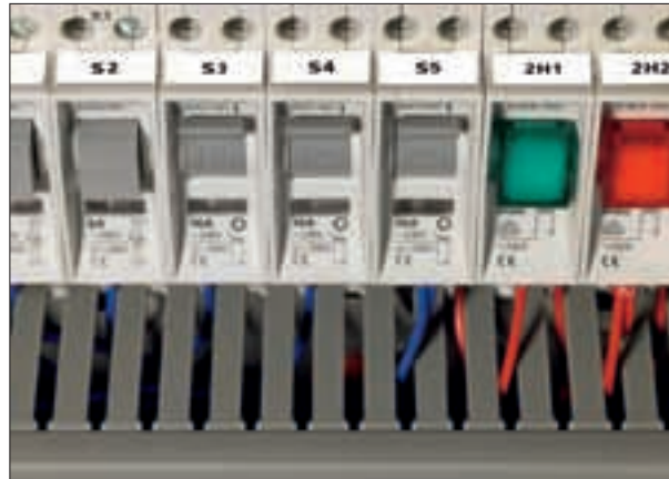
Clearly identified labels ensure easy network wire and cable management.
