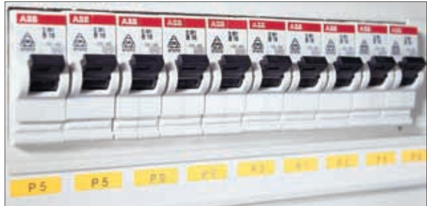
Helatag 860 switchgear application.
